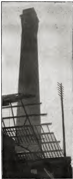
The chimney on which Esau Mayall was working when he met with the terrible experience here related.
